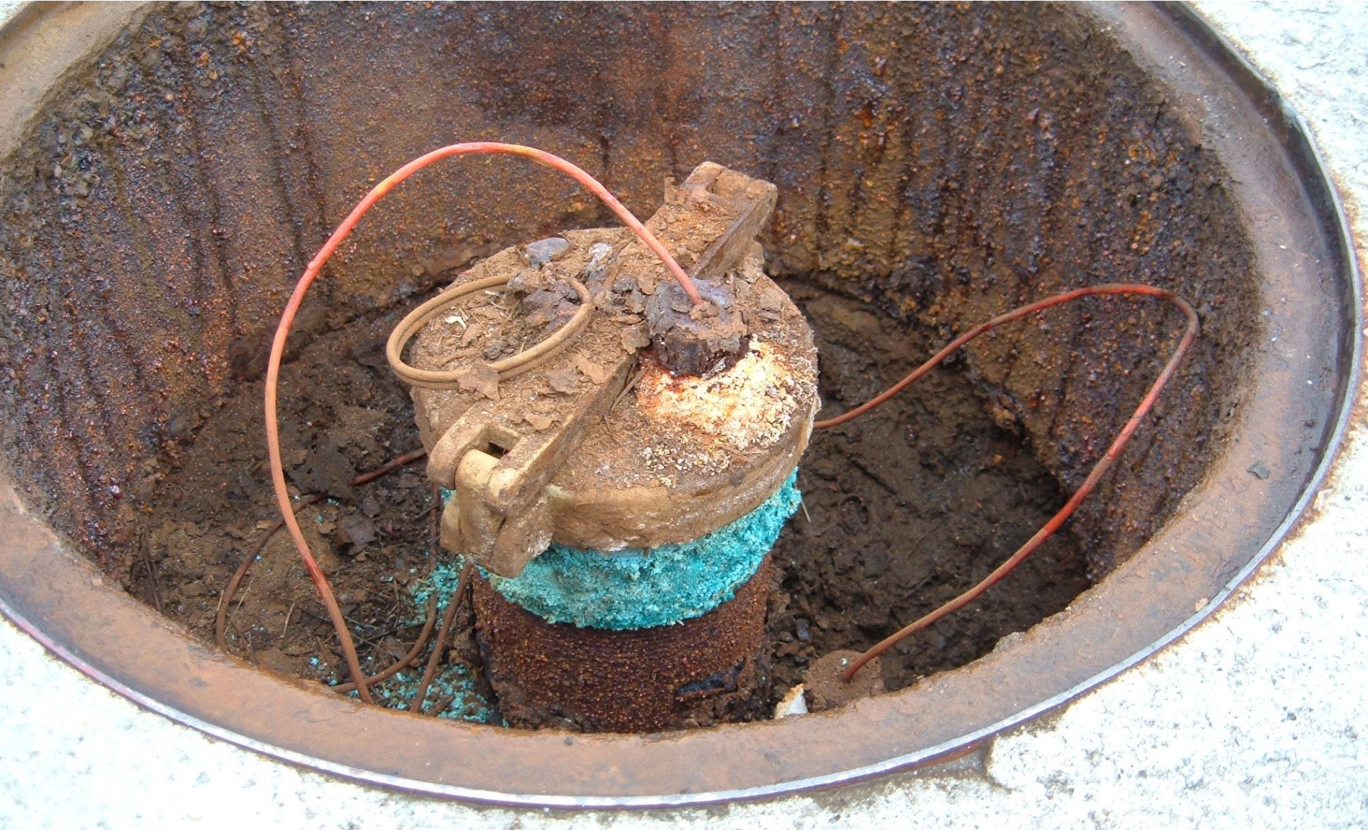
Evidence of vapor leaks
